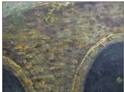
Figure 37: Sigmoid crack on the bridge (photograph by Hannes Elsenbroek)
